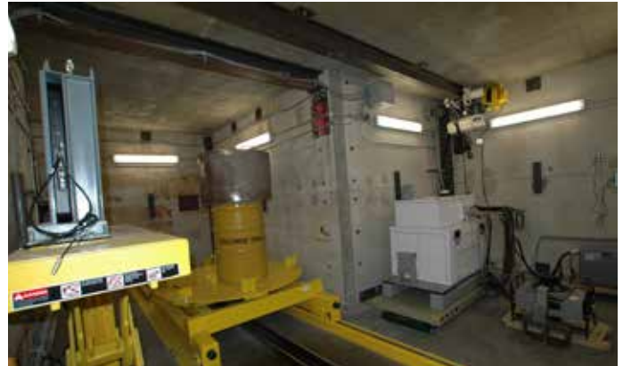
High Energy Vault
